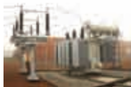
Pole transformatora 110/15 kV-16MVA 110/15 kV-16MVA transformer bay
